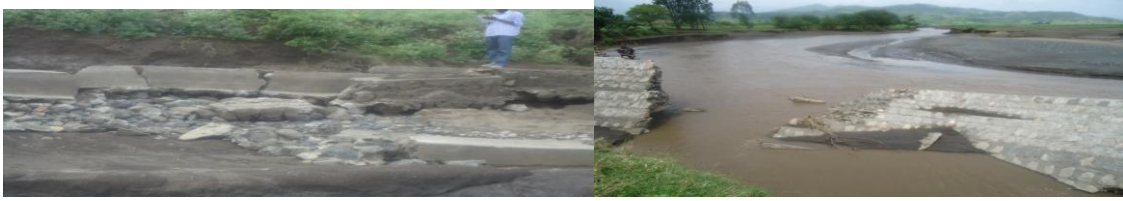
Fig. 10. Collapse of Gotu scheme by flood from the untreated catchment, North wollo
