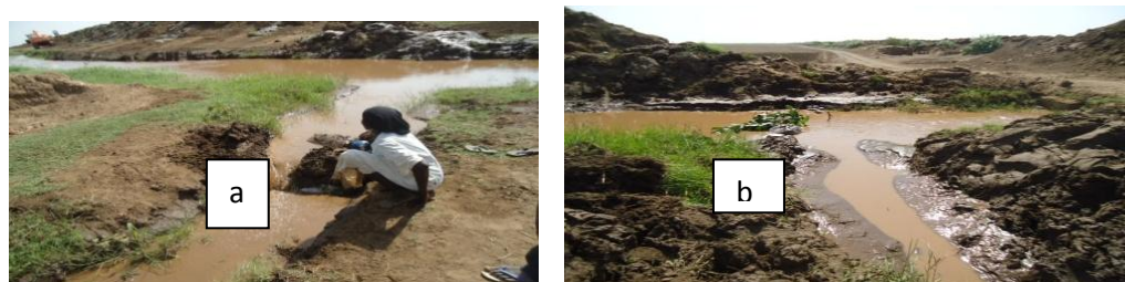
Figure 6. Water distribution difference because of absence of sediment management practice - on FOP 1 at Gezira Scheme. N.B. The first plate (a) shows in FOP1 water was flowing out over the suck-mud and this was most often the case before canal excavation. Plate (b) shows, after canal excavation, the amount of water discharging into this Abu XX decreased dramatically, so that farmers create a head across the minor.
